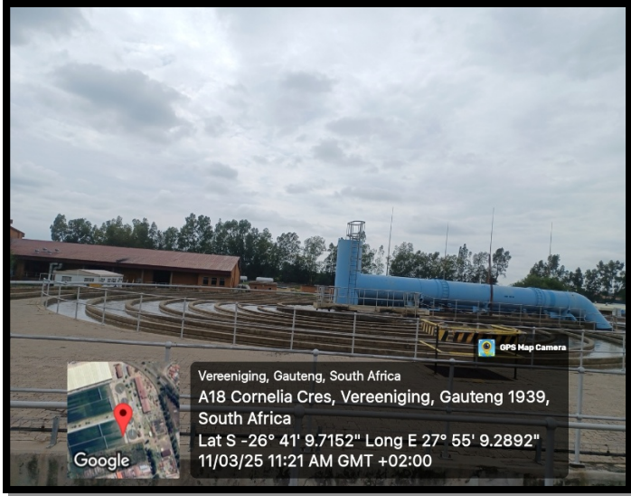
Figure 5: Flocculators for existing systems next to the proposed new system 1
